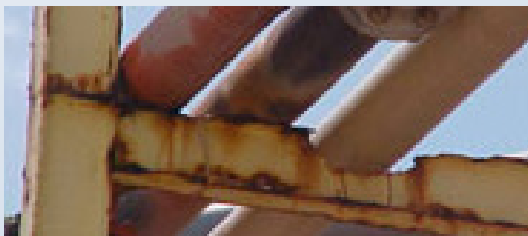
Pipe conditions without APS Raq-Gard®
